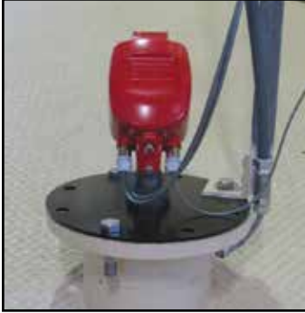
Actual installation in beverage industry.
