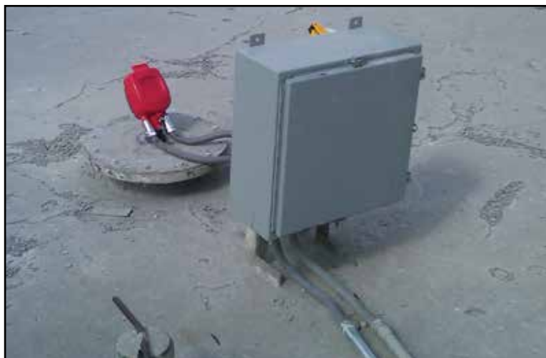
A dusty application in a cement plant.
